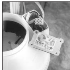
Romex wiring - Top View
